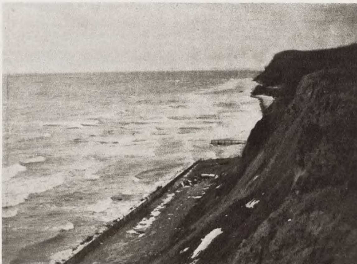
THE CONSTRUCTION OF A PROMENADE ON THE POLISH COAST NEAR GDYNIA (PHOT. S. PLATER)
